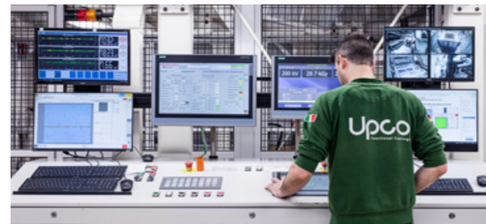
Upco line control panel
